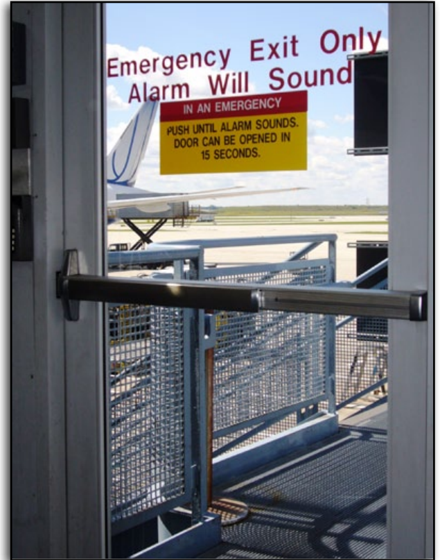
This exit door is part of a “delayed egress” system.
